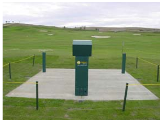
4View Installation, Poppy Ridge Rear View
